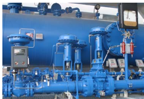
Three Phase Test Separator
