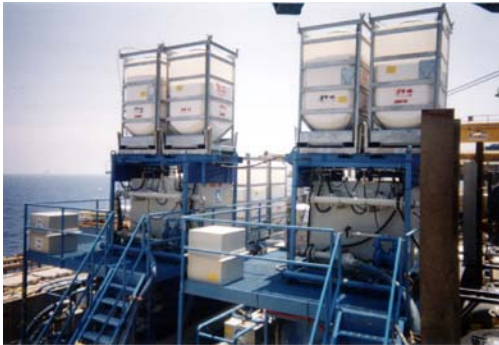
SafeDEflo System Installed on DE Mixing Skids During Offshore Filtration Operation
