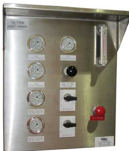
Emergency Shutdown Panel
